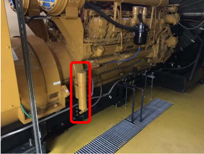
Genset with existing block heater (circled in red)
