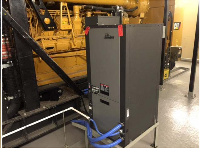
Sample genset with engine block heat pump installed
